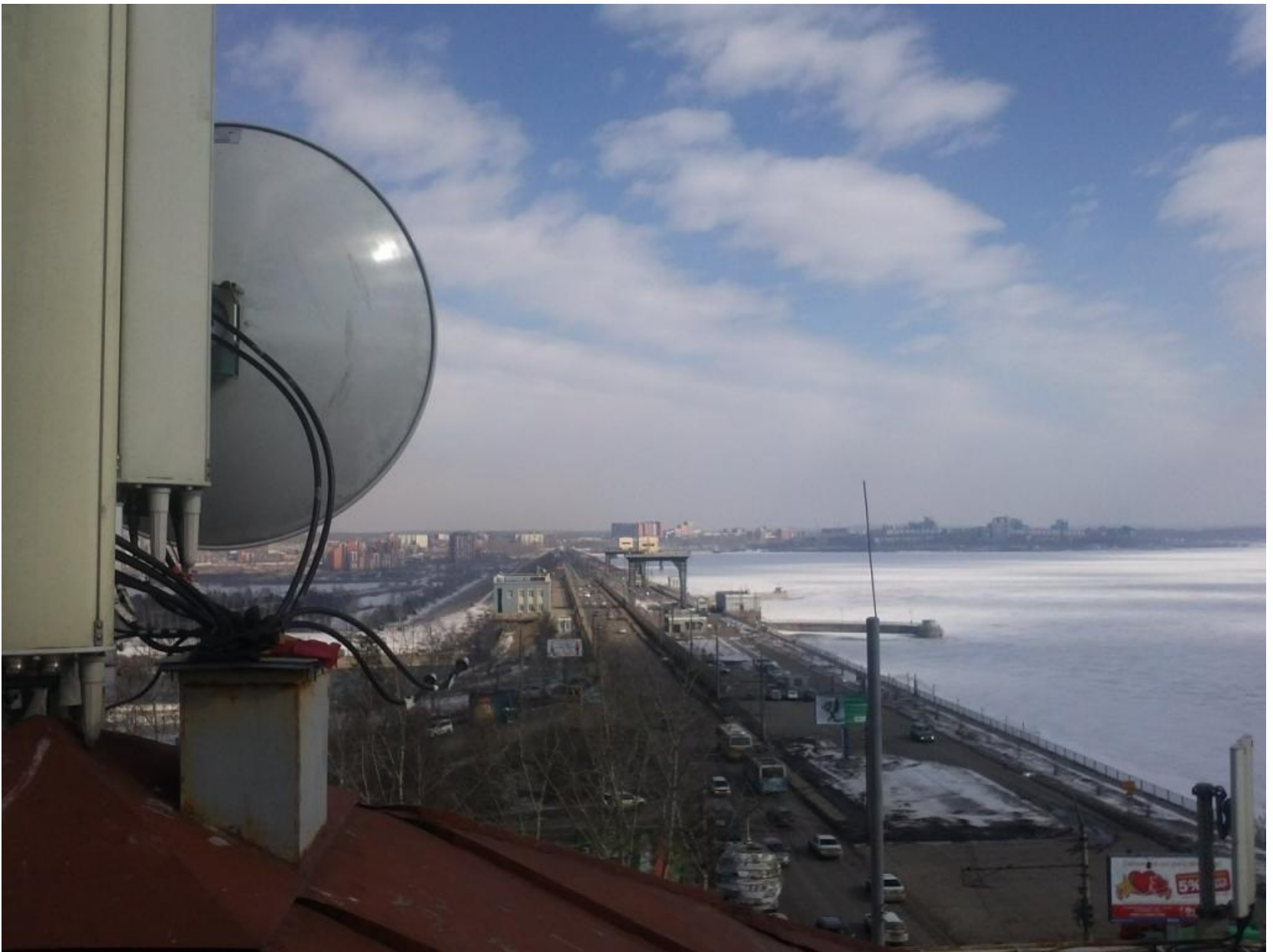
VEGA Mx CMP12 illuminating Long Bridge for Dominant Signal
